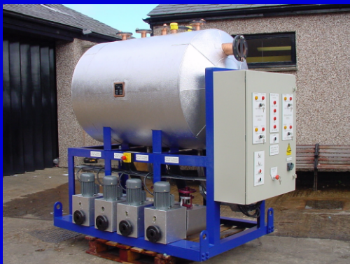
Condensate pump return set with BMS, level & temperature control for BNFL.
